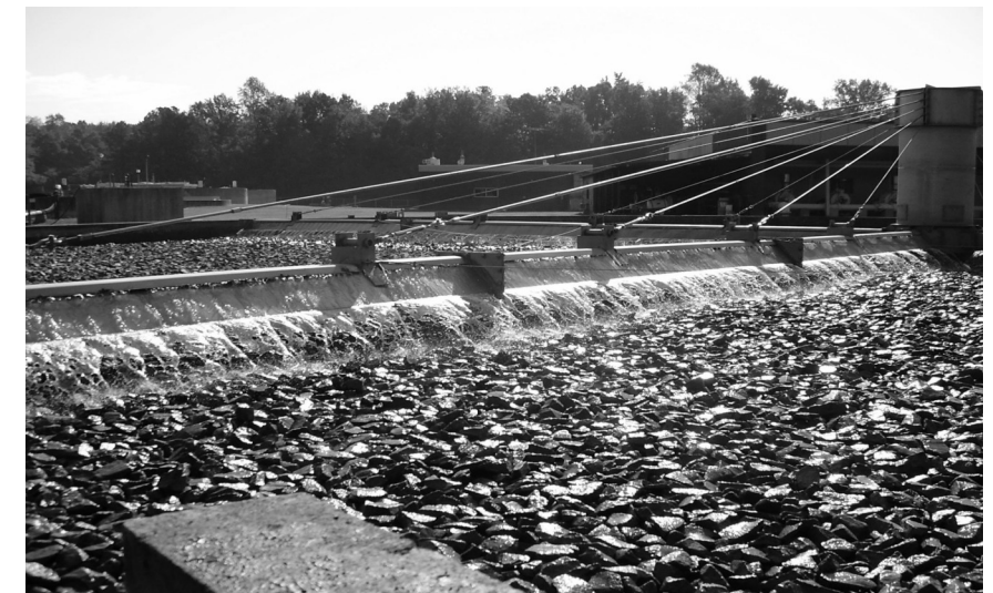
Rotary Distributor: First phase of secondary treatment
