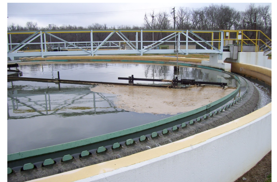
Illegal Grease Discharge
