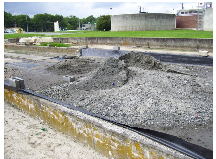
Debris from I/I as a result of Hurricane Andrea
